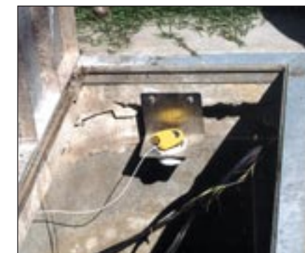
Municipal Pump Lift Stations
