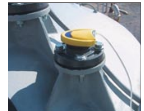
Chemical Bulk Storage Tanks
